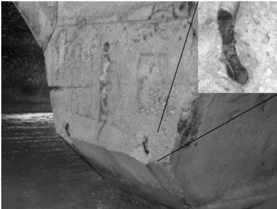
Girder No. 9, where most of the tests were performed. SCC occurred on rebar exposed at this girder.
